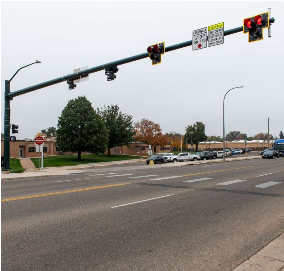
Pedestrian Hybrid Beacon Crossing
