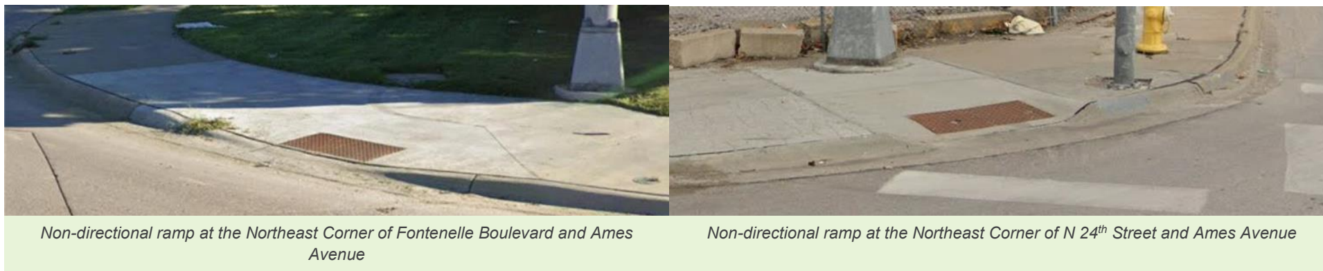
Figure 14: Examples of Non-ADA Compliant Ramps along Ames Avenue
