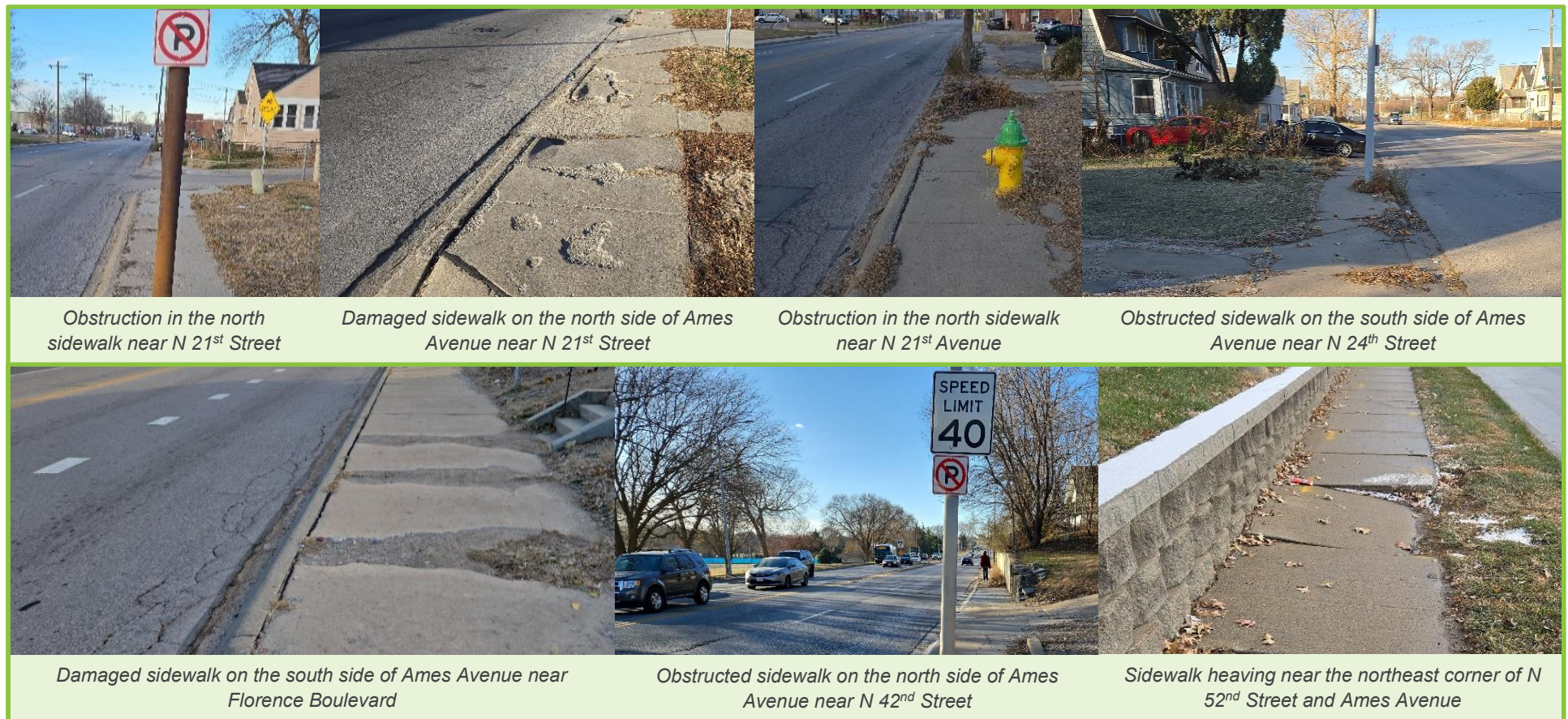
Figure 12: Examples of Sidewalk Deficiencies along Ames Avenue
